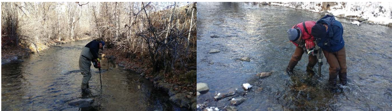
Figure 3: A) loosening the bed sediments with the hammer drill, B) installing the driver sleeve with the post driver.
