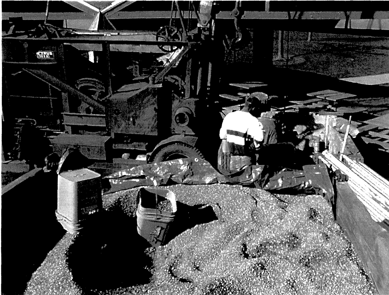
Gravel Pack Material in Dump Truck (pipe to the right is tremie pipe)
