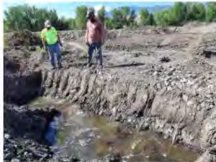
STAGE 1: MUD SLURRY IN BOTTOM OF EXCAVATED TRENCH WITH LIVE CUTTINGS PLACED WITH BOTTOM END EXTENDING BELOW GROUNDWATER.
