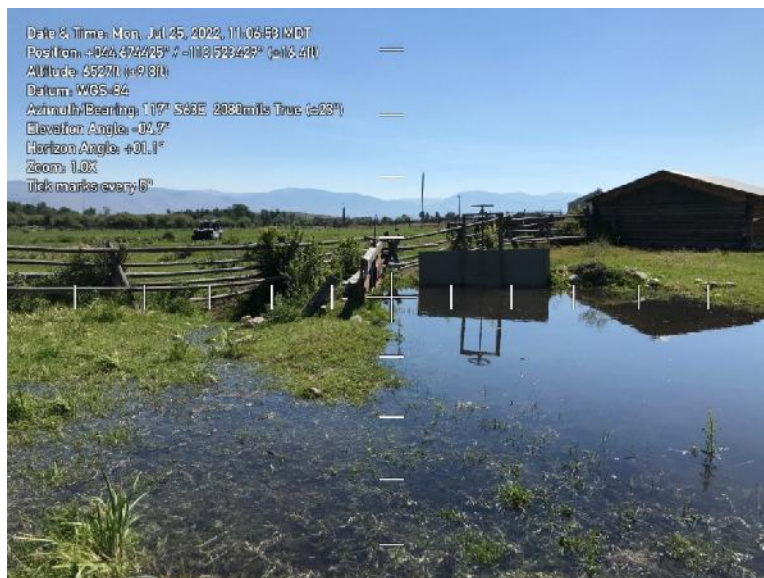
Photo 3. Water bypassing the Check Structure. The camera was facing approximately east from near Point C.
