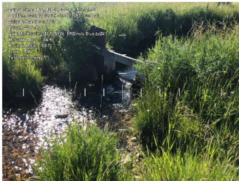
Photo 7. Cipolletti weir at Point G. The camera is facing approximately east.
