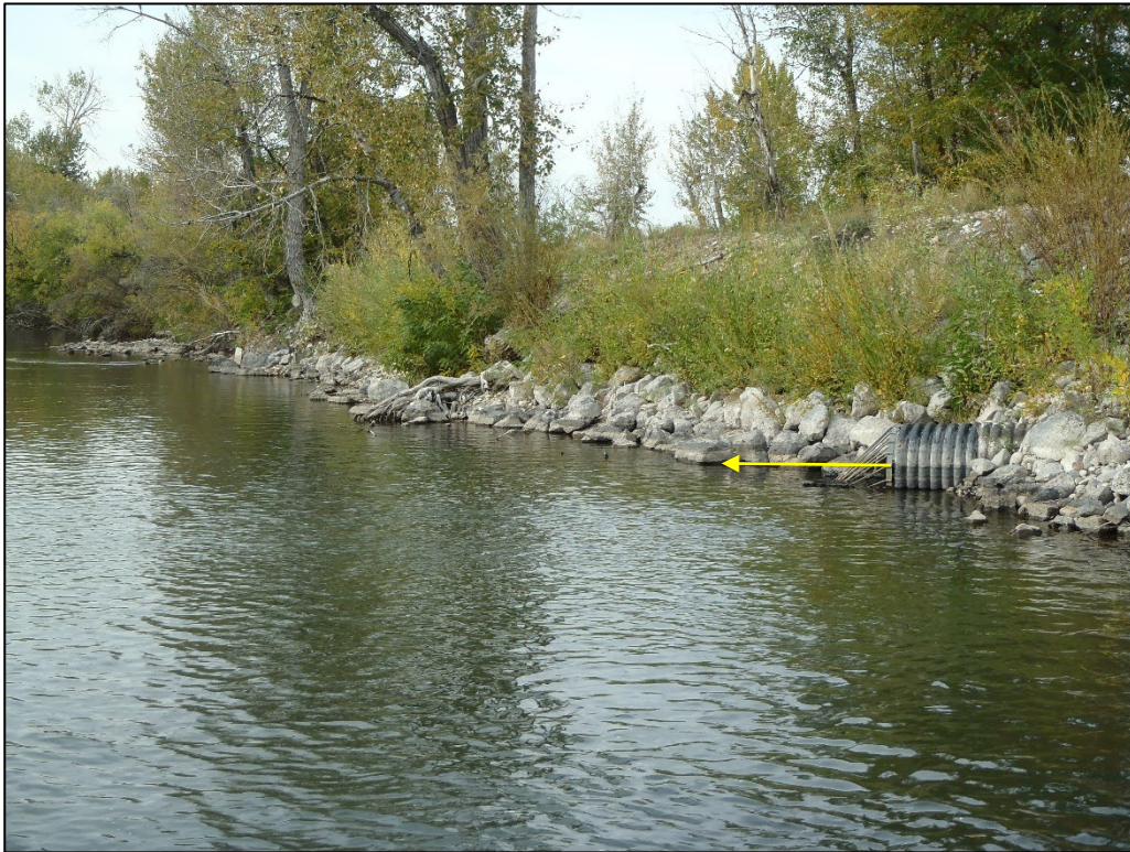
Photograph 10. Temporary Diversion Pipe Outlet to Boise River below Drop Structure 3 (October 2023).
