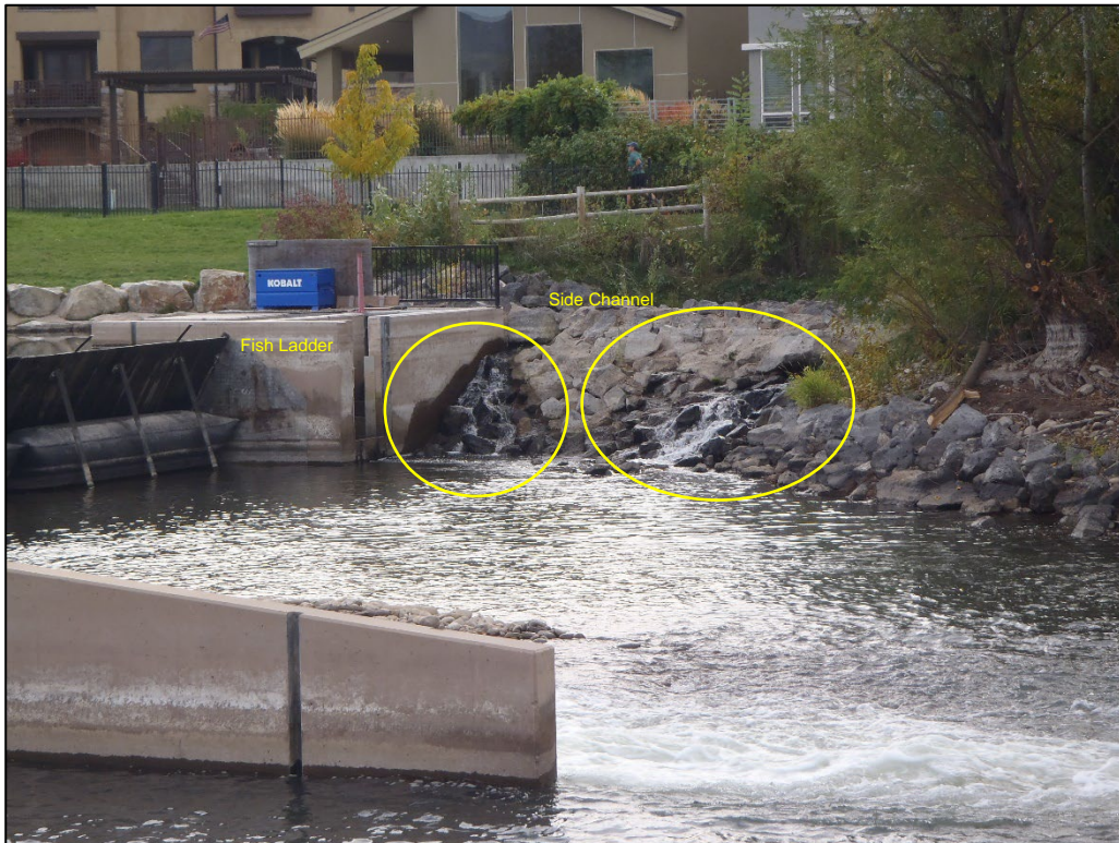
Photograph 4. Left Bank Side Channel Leakage Through Riprap and Grout (October 2023).
