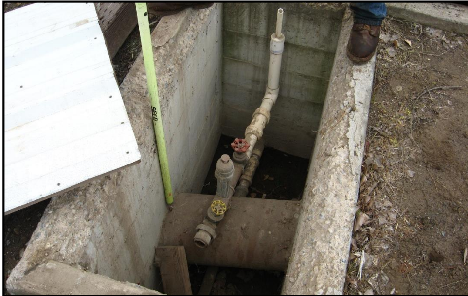
Photo 4. 14-inch pipeline exposed in vault.
