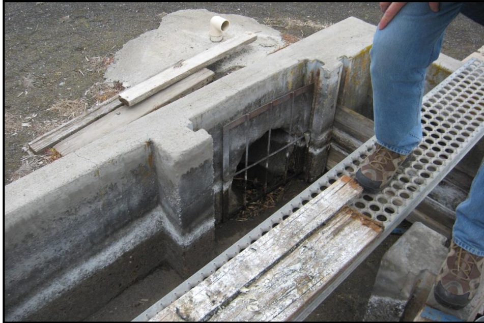
Photo 7. 18-inch pipeline at downstream end of small raceways
