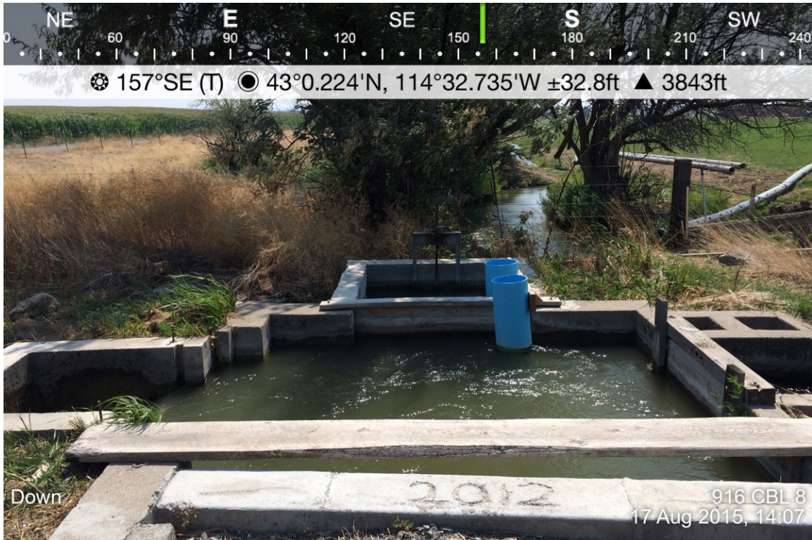
1. 916CBL8 diversion, directly south is the submerged orifice. Water comes from under the road heading south, to the left (east) is 916CBL End, to the right (west) 916CBL9.
