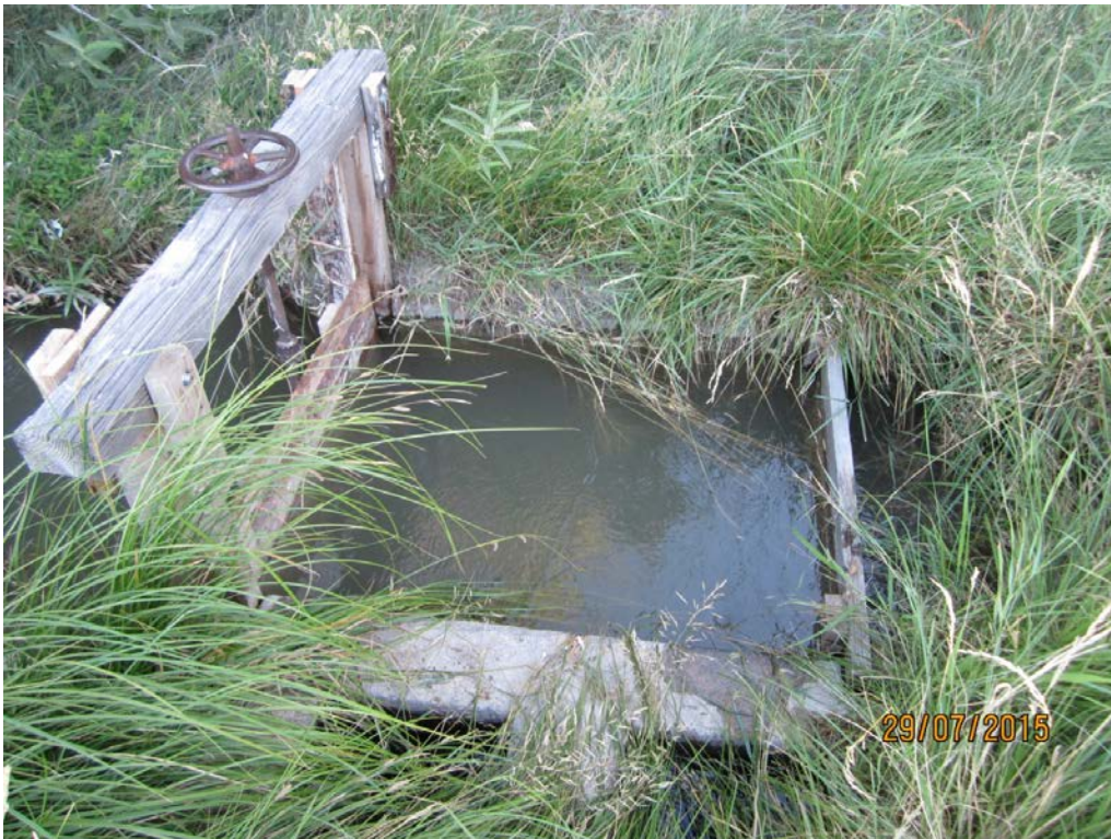
2. Mabbut 70Ditch: orifice-control gate box.
