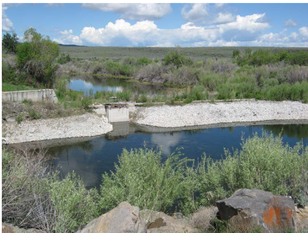
1. Richfield Canal: concrete diversion dam across river with gravel/dirt pushed-up along upstream face of dam. Concrete box and control gate for flow release and control is located near bank on left side of photo (view of river looking downstream).
