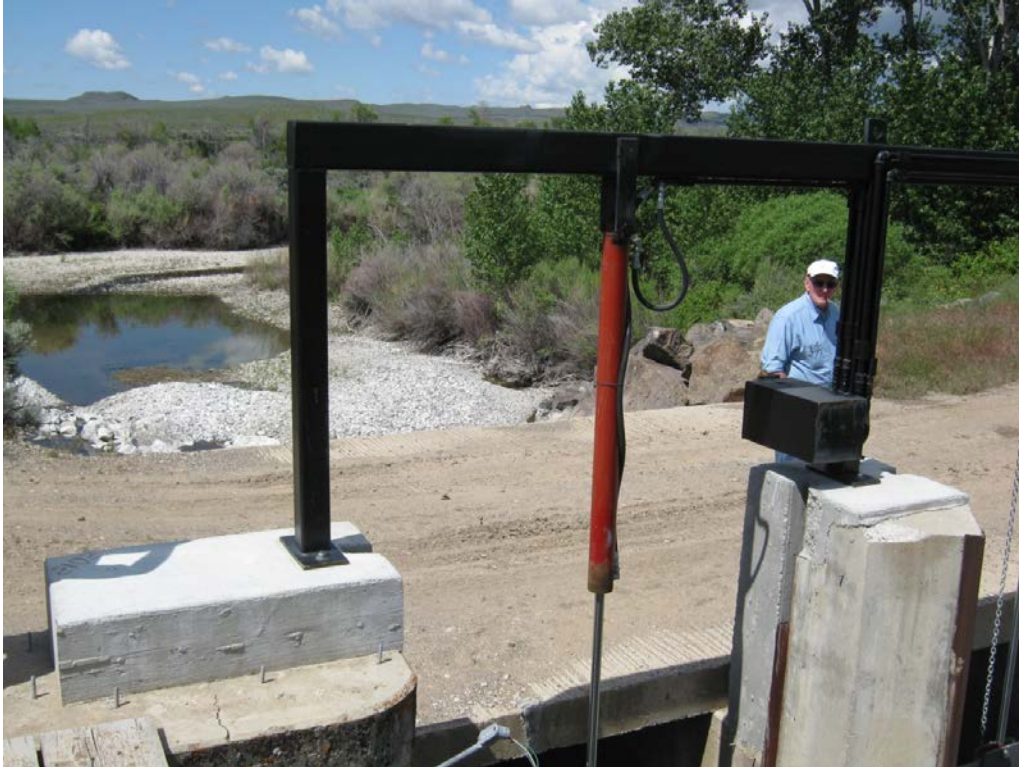
5. Richfield Canal: Spill gates in foreground, water spills to Big Wood River In background.
