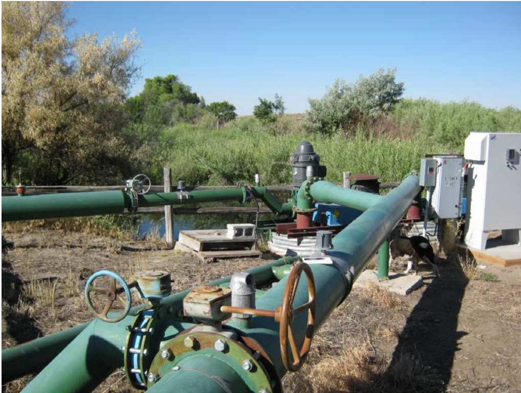
1. Oppio pumps: small pond from river in background to pipe intake/sump on left with 50 HP pump in background connected to 8" mainline. A 14" mainline in foreground from sump and 15 HP centrifugal pump on right. Note flow meter on 14" mainline.
