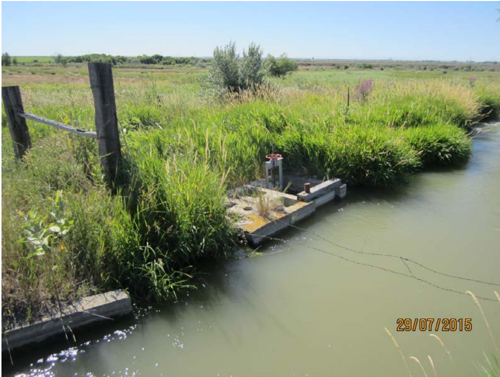
1. Union Ditch 27 Lenguineche re-diversion head gate, orifice – head gate control box. Water diverted to open ditch and flood irrigation system.
