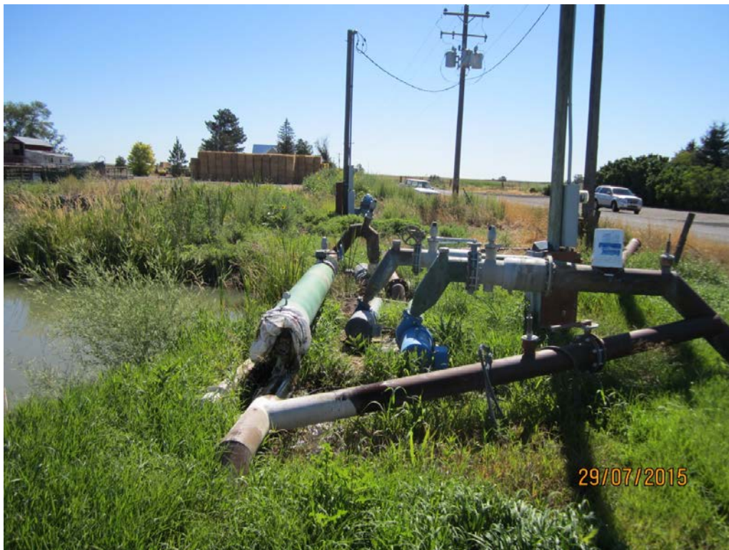
4. Pond and three centrifugal re-lift pumps to irrigation system. Well located behind utility pole is tied into same irrigation conveyance system.
