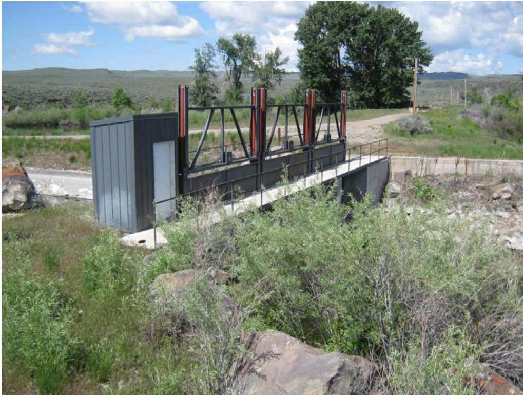
2. Richfield Canal: hydraulic canal gates in concrete abutments at head of canal next to diversion dam across river.
