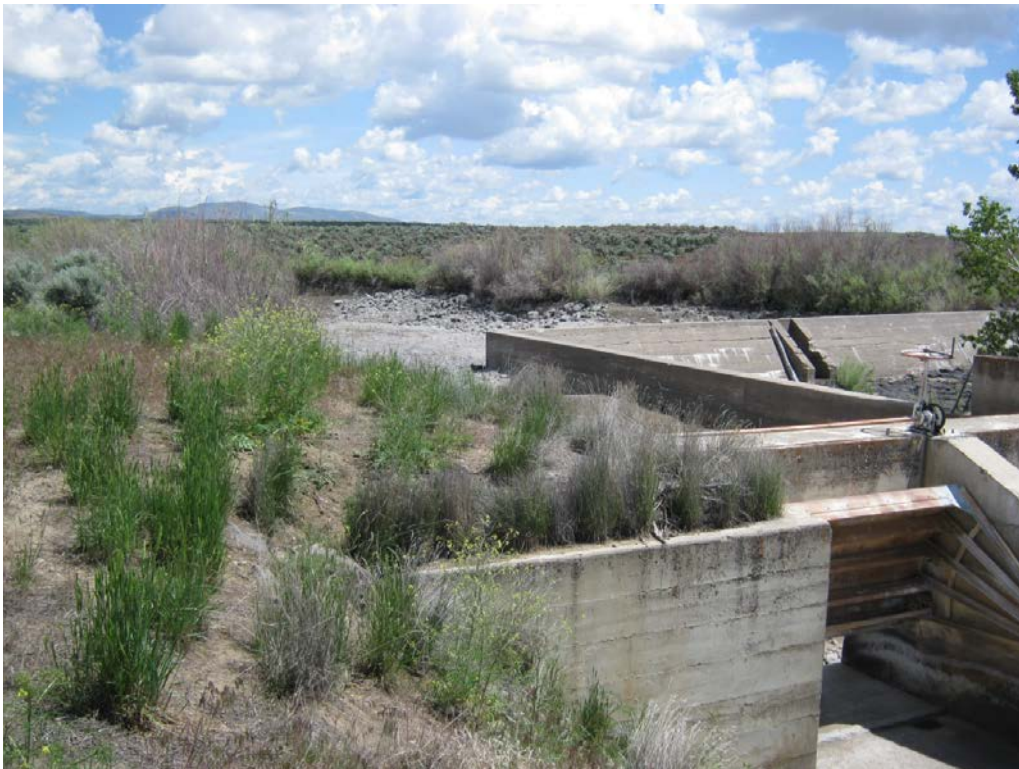
2. View of dam, river channel, and left end of head gate structure with radial gate.
