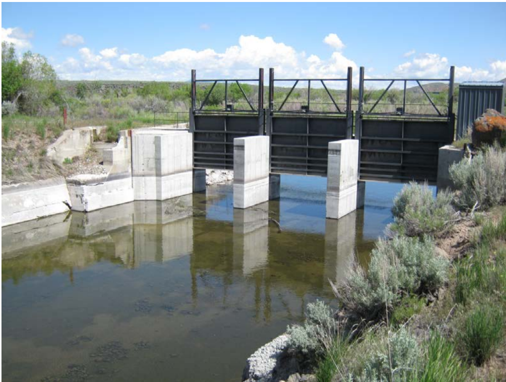
3. Richfield Canal: downstream view of main canal gates next to river diversion dam.
