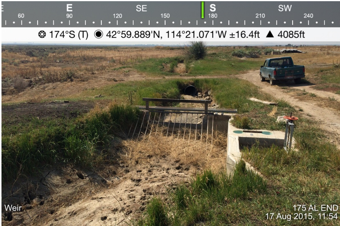
1. Downstream view of 175AL End weir blade; to the right is a submerged orifice and screw top head gate for separate diversion for different user.
