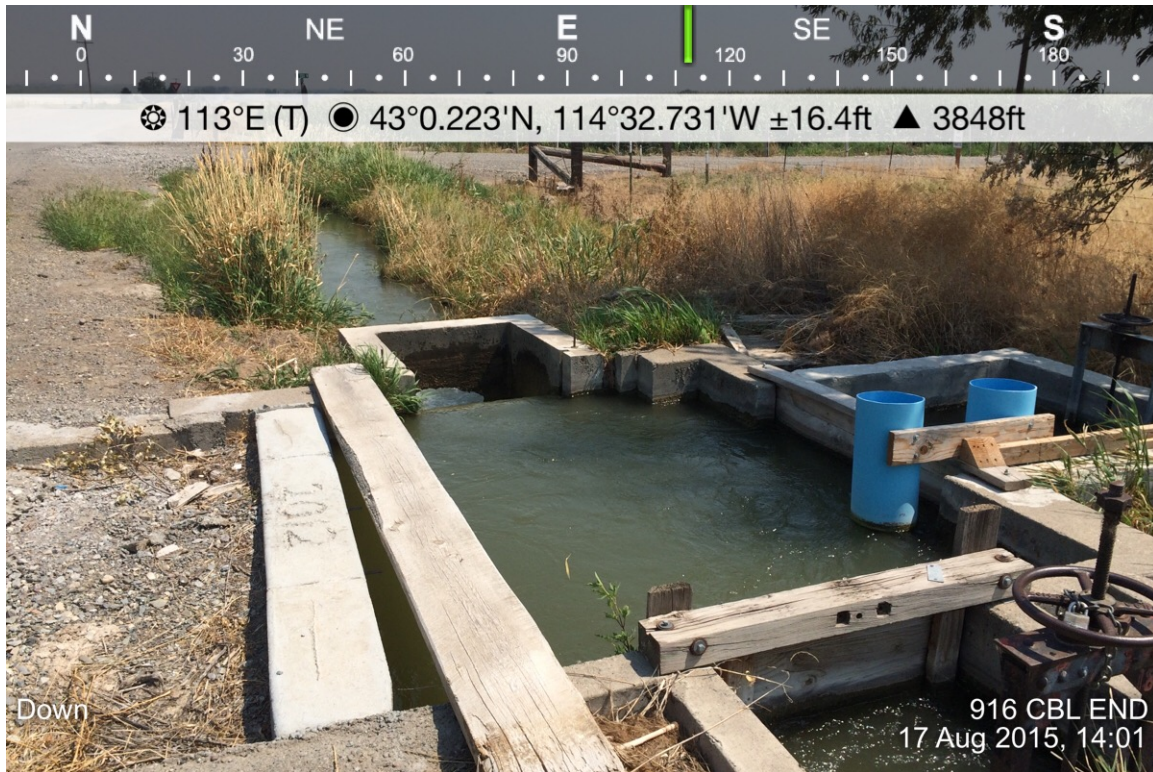
1. Ritter Pump 66: intake pipe from river to pump.
