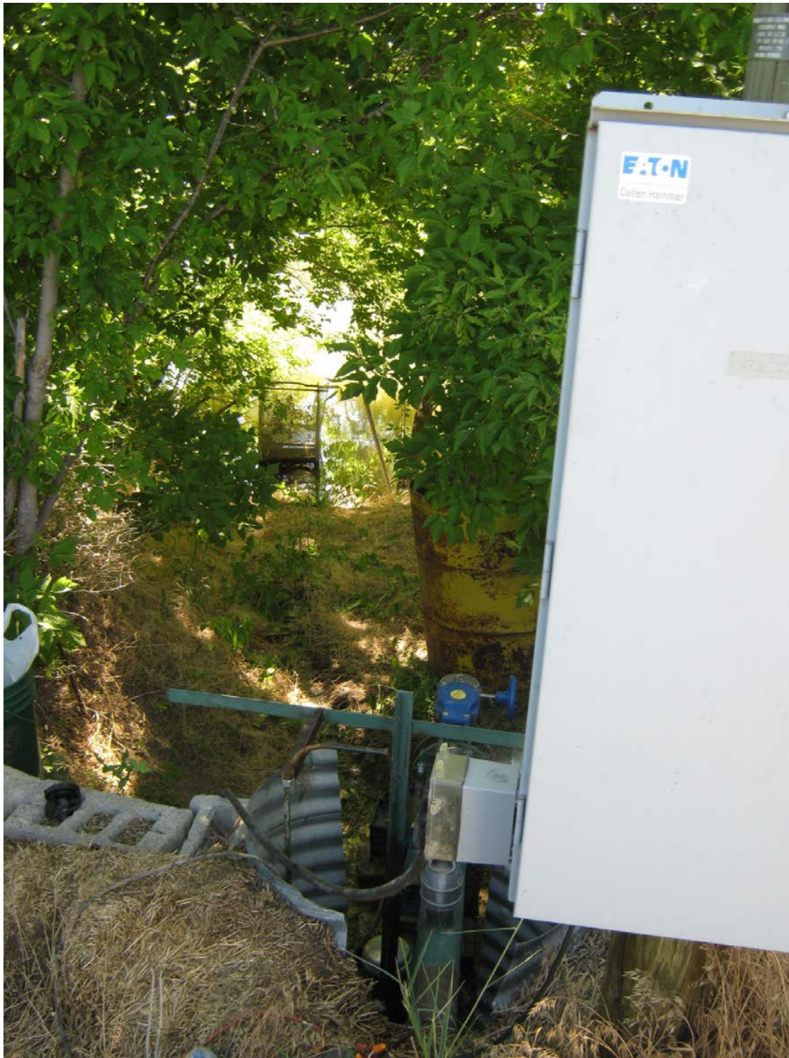
1. Small size centrifugal pump in CMP sump to 4" mainline. Intake pipe from river (in background to sump).
