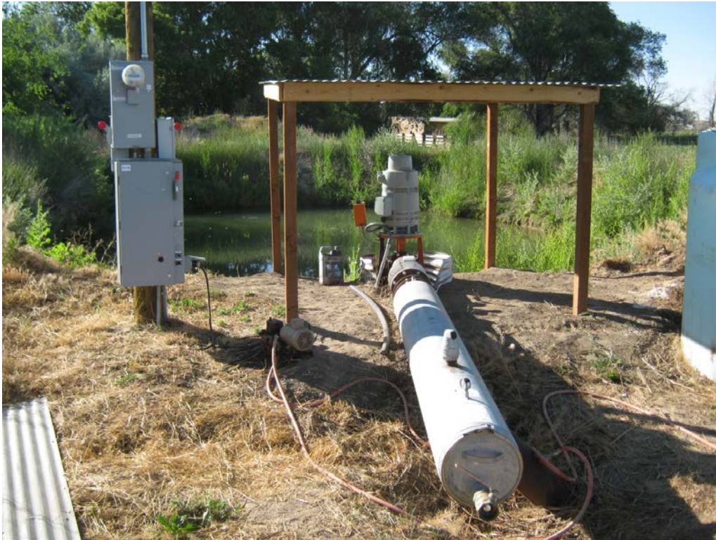
1. Hults pump or Jones 35-P4A: 25 HP pump in CMP sump from pond off river. Mainline to dragon filter, and mainline off filter to irrigation discharge points - pivots and corner hand lines.
