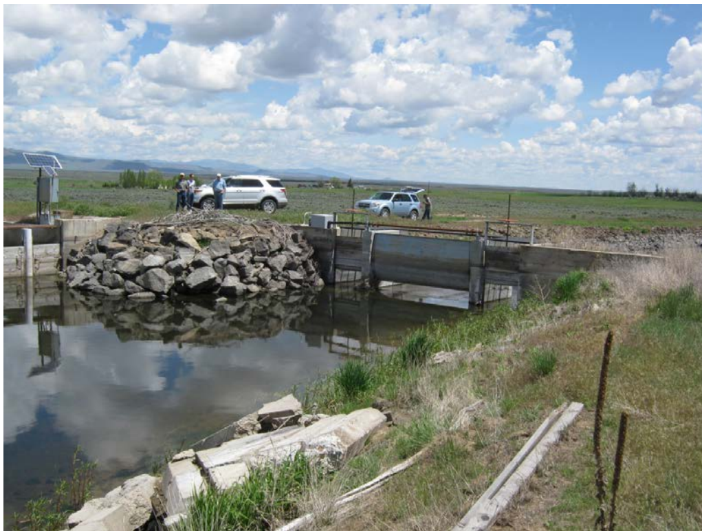
11. Richfield Canal split BWCC East and West Main Canals (head gate control structure on right), and Jim Byrns Slough (head gate control structure on left side of photo).
