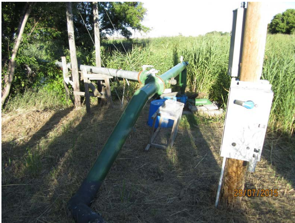
4. Mabbut 70P: 20 HP pump from wet well, to mainlines and sprinkler systems.
