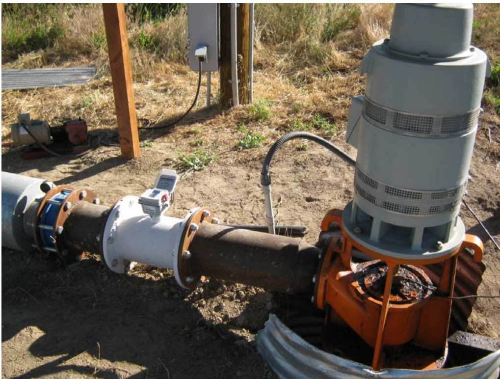
2. View of sump, pump, and 8" mainline with Seametrics mag meter.
