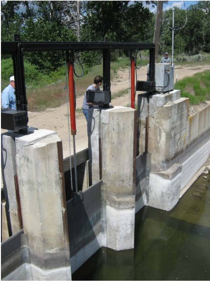
6. Richfield Canal hydraulic spillway slide gates.
