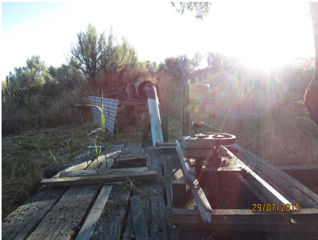
2. Mabbut &0-P: Viev of 5HP pump from river side, looking at mainline to ditch in background.
