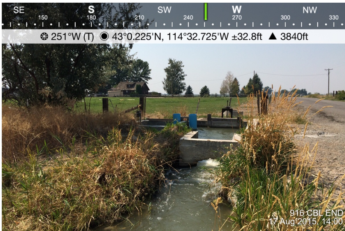
2. Ritter Pump 66: CMP well to vertical turbine 50 HP pump, connected to dragon filter (background, left) and mainline (right, with 10 inch Mag meter).
