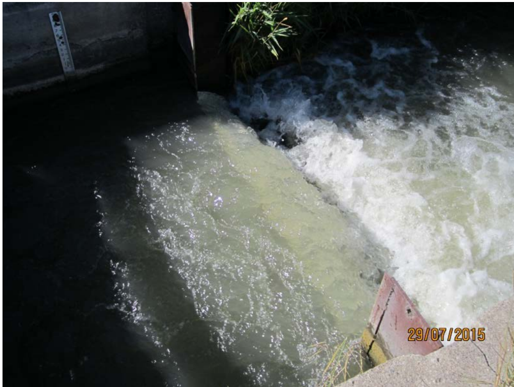
3. Rectangular weir in head gate control box, about 7' below gate. Note high approach velocity and turbulence.
