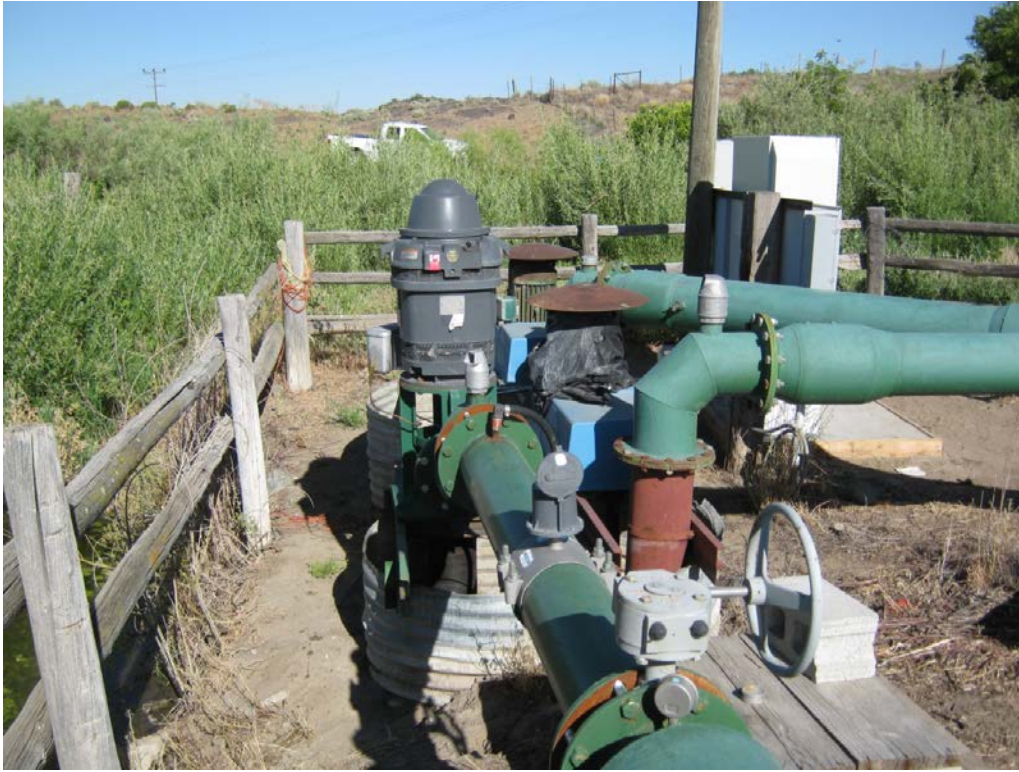
3. Pumps from CMP sumps connected to mainlines. Middle centrifugal pump did not appear to be in use. Note McCrometer flow meter on 8" mainline from 50 HP pump.
