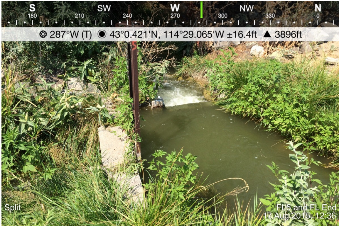
1. FL End weir, to the left of the weir is the FL5 head gate.
