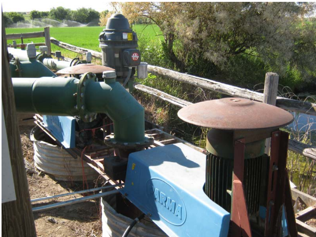
2. Sump on right with 15 HP centrifugal pump (right) to 14 inch mainline.
