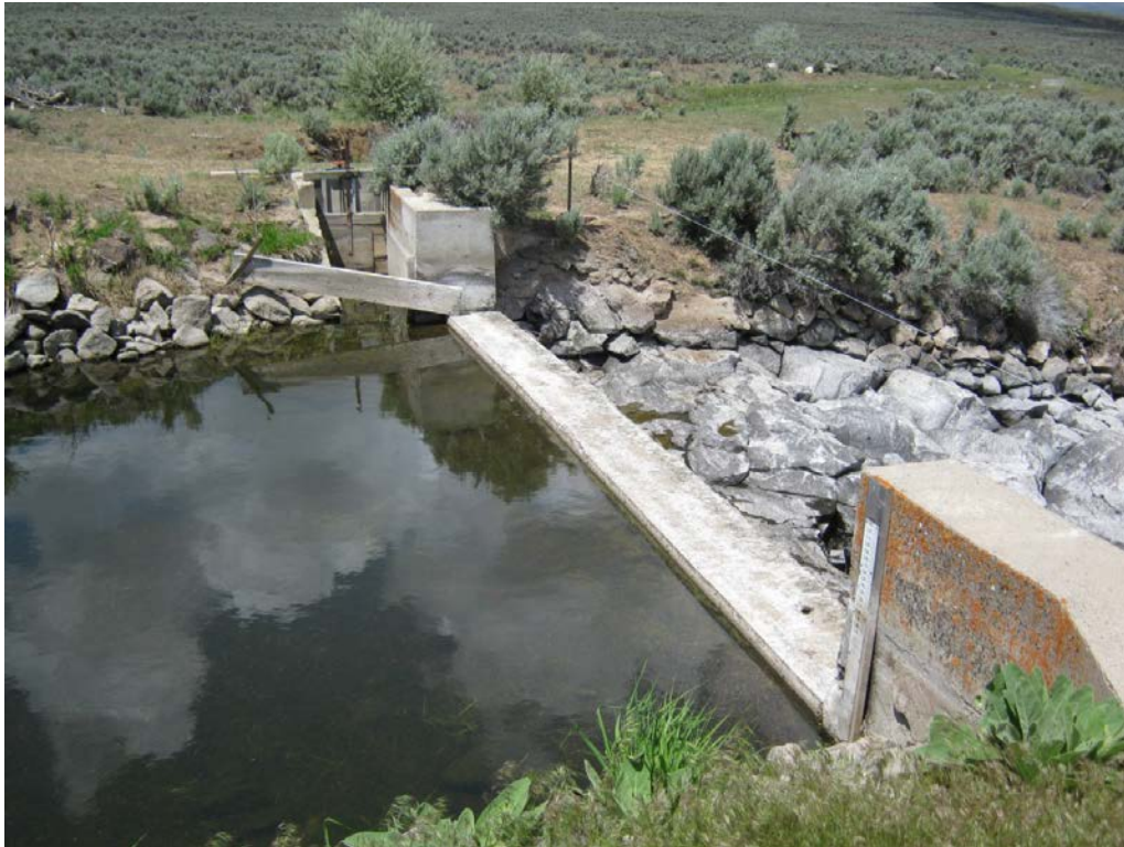
13. Jim Byrns Slough measuring device and staff gage. Check dam type structure used as standard contracted rectangular weir (28 ft. width). Note head gate to small ditch next to weir (top – center of photo).
