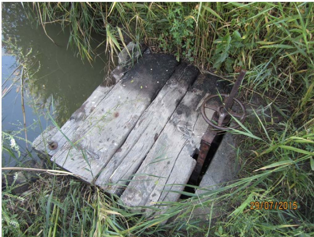
6. Mabutt 70P: Diversion box in river that diverts water to wet well with pump. Submerged orifice on front/riverside of box and slide gate with hand wheel on ditch discharge side for control.
