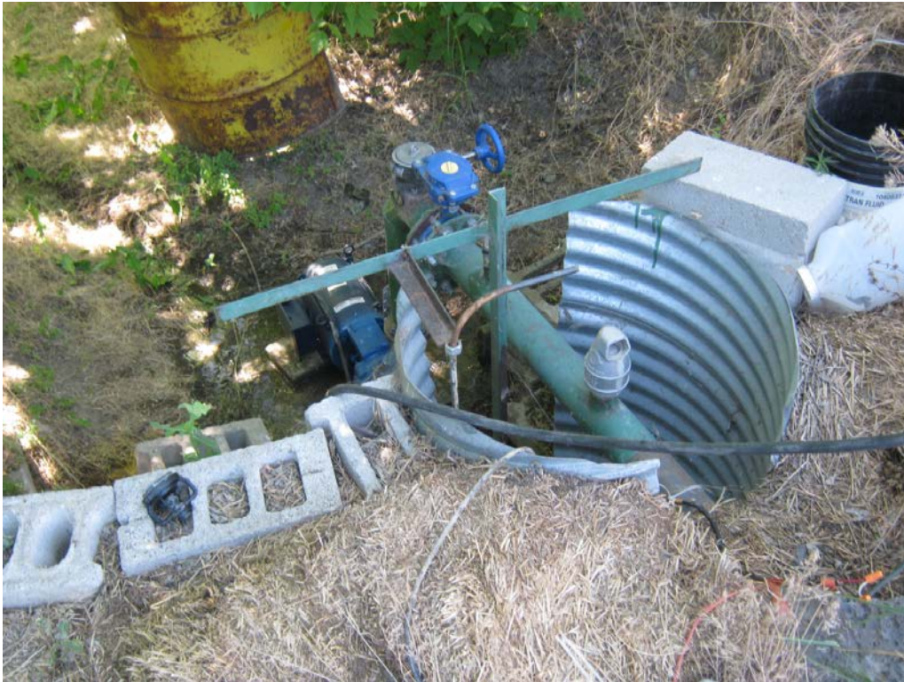
2. Close-up view of sump and pump.
