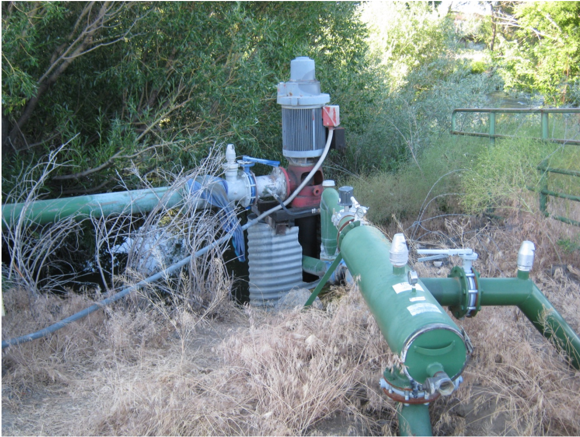
1. Desert Rose pump: 15 HP centrifugal pump (on right, view partially blocked by filter) to 6" mainline, dragon filter and mainline off filter (on right hand side of photo). McCrometer meter on 6" mainline above dragon filter. Faulkner pump on left shares same CMP wet well/sump.
