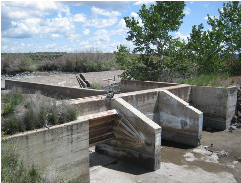
1. Lincoln Bypass diversion dam (background) and control gate structure (foreground). Three gate bays with one radial gate on left end, other bays are concrete sealed.
