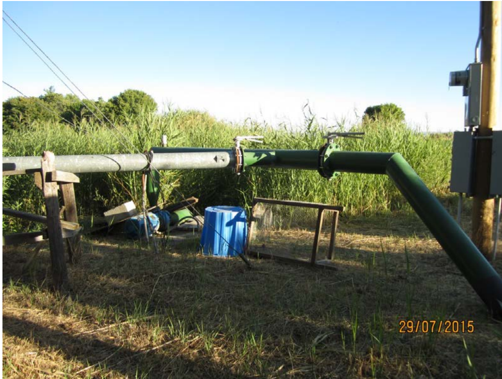
5. Mabutt 70P: 20 HP pump to discharge pipe that splits to two mainlines.
