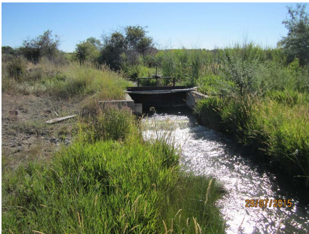
2. Robertson Ditch, head gate control structure with rectangular weir.
