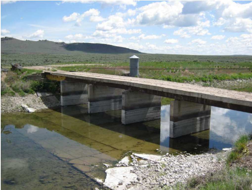
8. Richfield Canal rated measurement section and station. Stilling well in background houses continuous recorder equipment.
