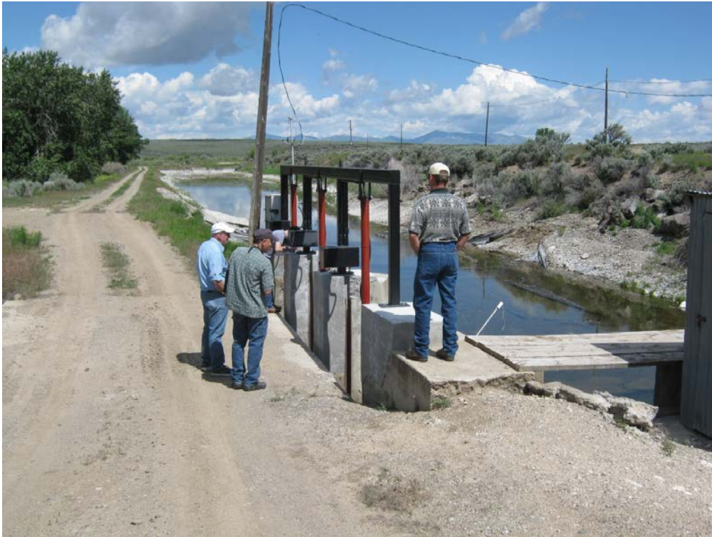
4. Richfield Canal: Spillway gates located on canal downstream of main canal gates and river diversion dam about 365 yards. Water spills to the Big Wood River (located to the left of the photo). Check structure across canal to the right.
