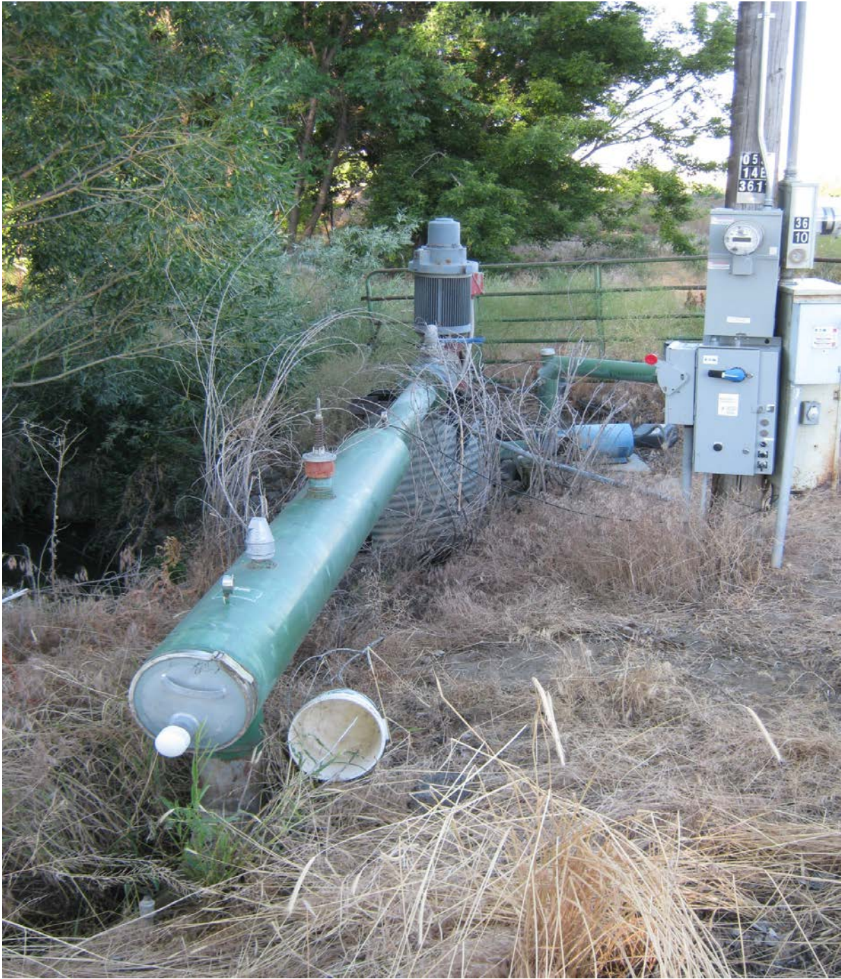
1. Faulkner-Bliss Point pump: pump/60 HP motor in background from sump to 8" mainline, dragon filter, and mainline off filter.
