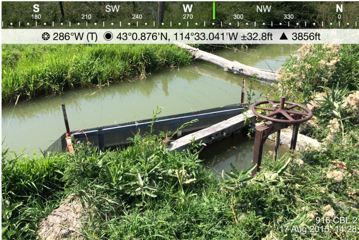
1. 916CBL 2 diversion and submerged orifice.
