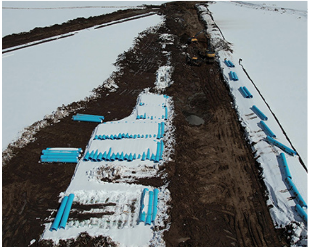
Tight window for construction requires trenching and pipeline placement when weather allows throughout the winter months. (Courtesy North Fremont Canal)
