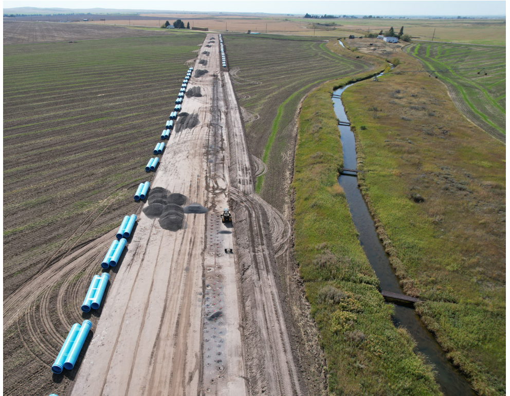
Phase 5 of the North Fremont Canal pipeline project getting under way in the fall of 2024. The project is the final phase of 20+ years of canal-improvement projects in the Ashton area. (Photo courtesy North Fremont Canal)
