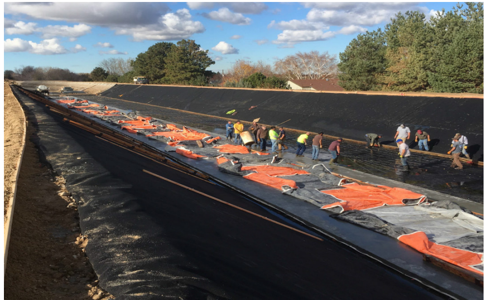
Rehabilitation work under way on the New York Canal. The geomembrane canal liner will be capped with concrete to complete construction. (courtesy Boise Project Board of Control)
