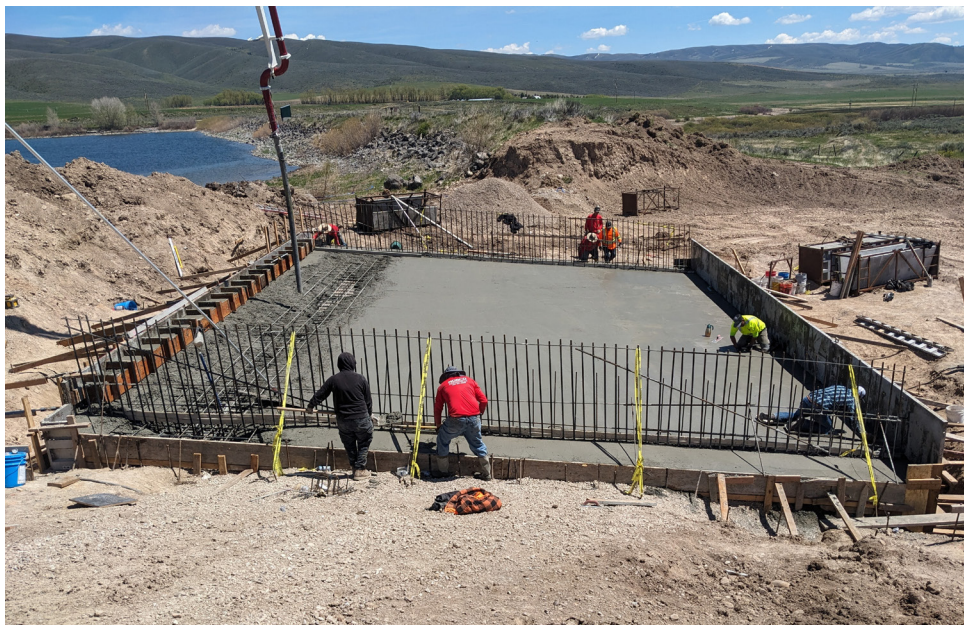
Contractors pour concrete pad for new spillway. A flood event in Spring 2023 undermined the safety and performance of the old spillway. (photo courtesy Portneuf Marsh Valley Canal Co.)
