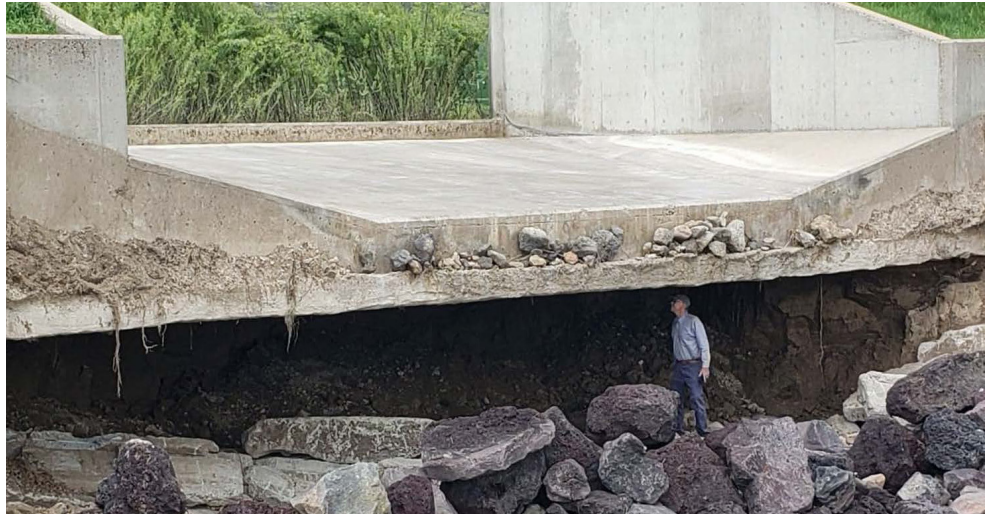
An Idaho Department of Water Resources safety engineer inspects the spillway damage following the 2023 flood event. (photo by Cindy Clark)
