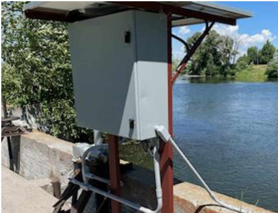
New headgate automation equipment installed on the Farmers Friend Canal in the Henrys Fork Basin (Courtesy Aaron Dalling/FMID).
