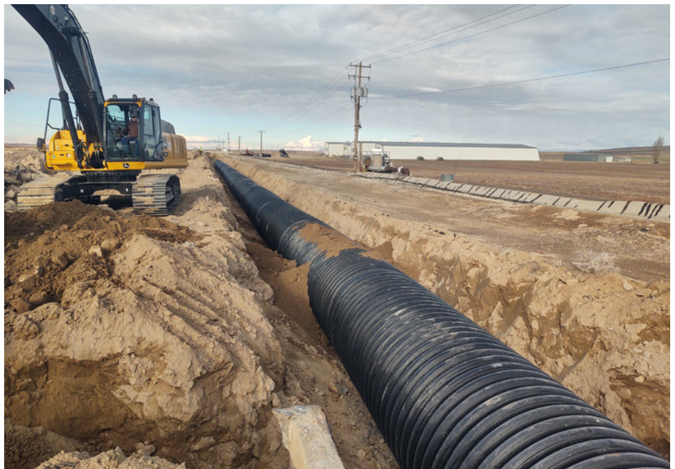
The Hat Butte Mutual Canal Co. converted a leaky old concrete open irrigation ditch to an enclosed pipeline with a $78,965 AIG, funded in 2022.
