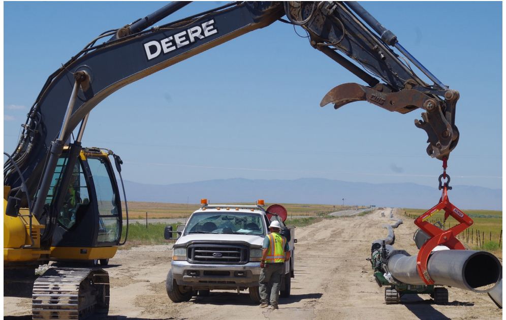
IMCO welds sections of HDPE pipe together along Idaho State Highway 167. The new pipeline will convey water to Mountain Home AFB. (photo by Steve Stuebner/IWRB)
