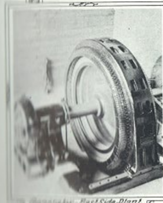
Generator - East Side Plant
