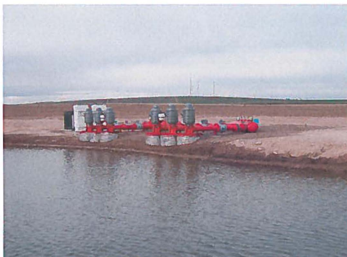
North Unit Pumping Station and Regulating Pond
