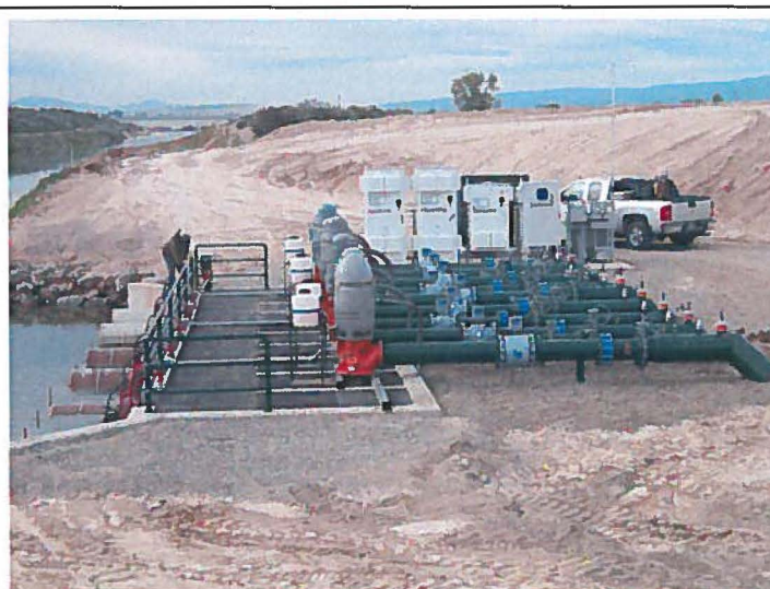
South Unit Pumping Station on North Side Canal
