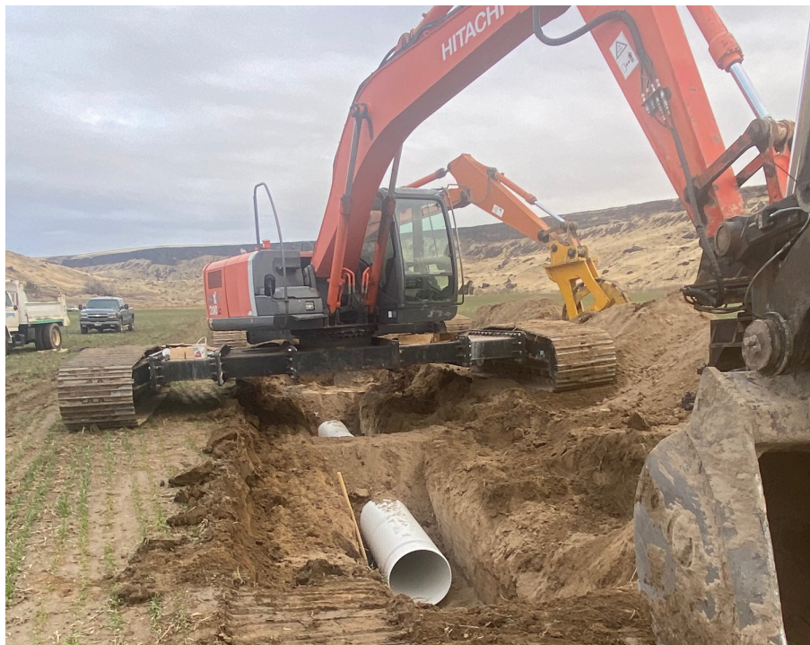
The Spinkler Shop Irrigation Co. installs new irrigation pipe in the West Indian Cove irrigation system. (photo by Dale Hooley)
