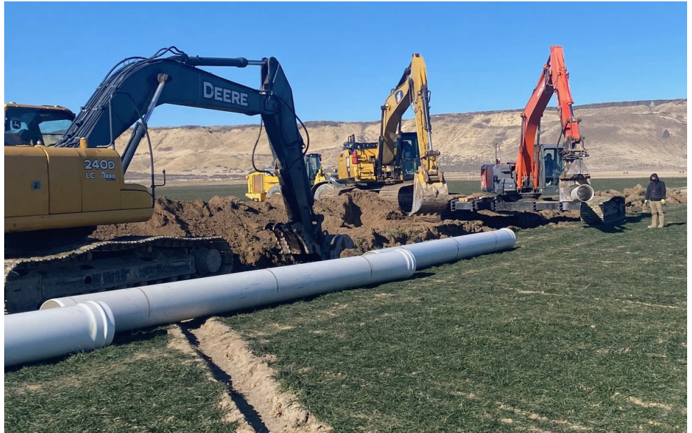
Trenches are dug and ready for new irrigation pipe to be installed. (photo by Dale Hooley)
