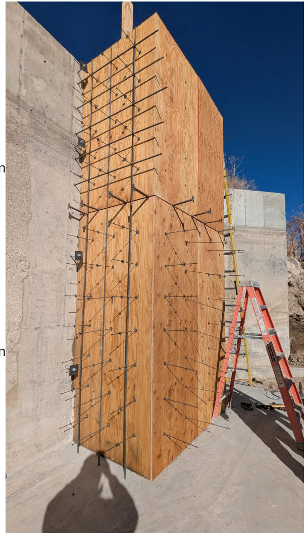
SlipMeter installed in existing concrete control structure near Hansen. (courtesy TFCC)
