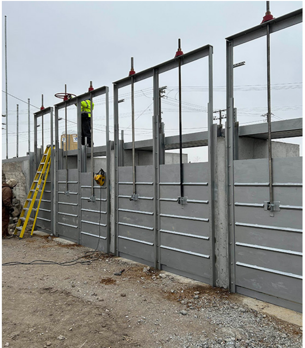
The new gates for the check structure are 6 feet tall. (Courtesy MID)
