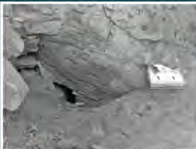
PS49-147-5173 NA Teton Dam, Teton Project, Idaho View of open joints on the right abutment at elevation 5133, station 15+30, 250 feet upstream. The joints are being separated. Morrison-Knudsen Company, Inc. and Peter Kiewit Sons' Company, Specifications No. DC-6910. 11/14/74 Bureau of Reclamation photo by B. Bockstruck
