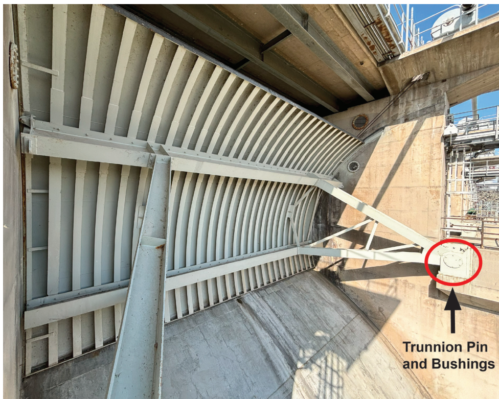
Close up view of a radial spillway gate on American Falls Dam shows the location of the Trunnion pin and bushing assembly at the pivot point of the gate. The old pins seized up over time, requiring replacement. (photo by Steve Stuebner/IWRB)
