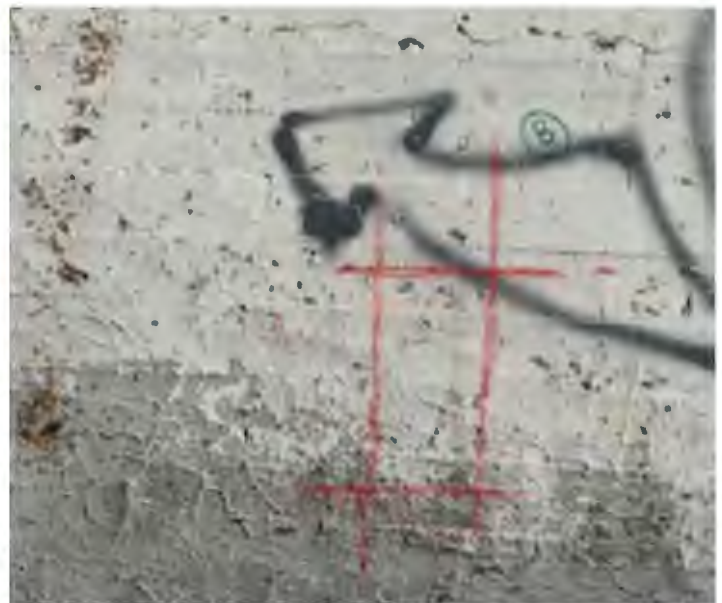
Location 8: Wall has vertical rebar at ~ 5 inches on center. Cannot "see" below this mat of rebar.
