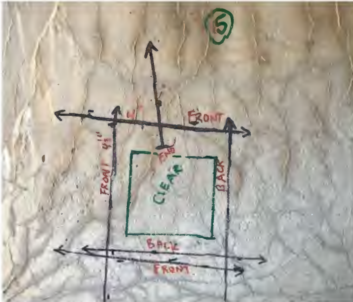
Location 5: Wall has a double mat of rebar that appears to be ~#4 bar.
