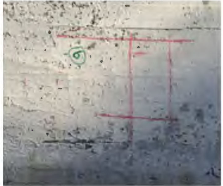
Location 6: Wall has vertical rebar at ~ 5 inches on center. Cannot "see" below this mat of rebar.
