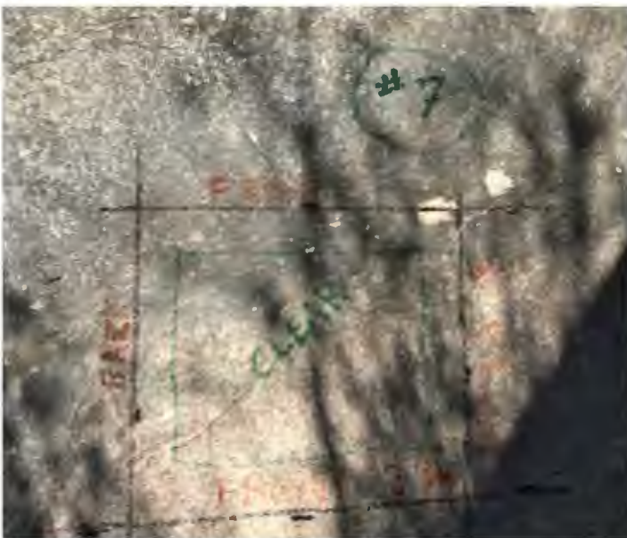
Location 7: Wall has a double mat of rebar that appears to be ~#4 bar.
