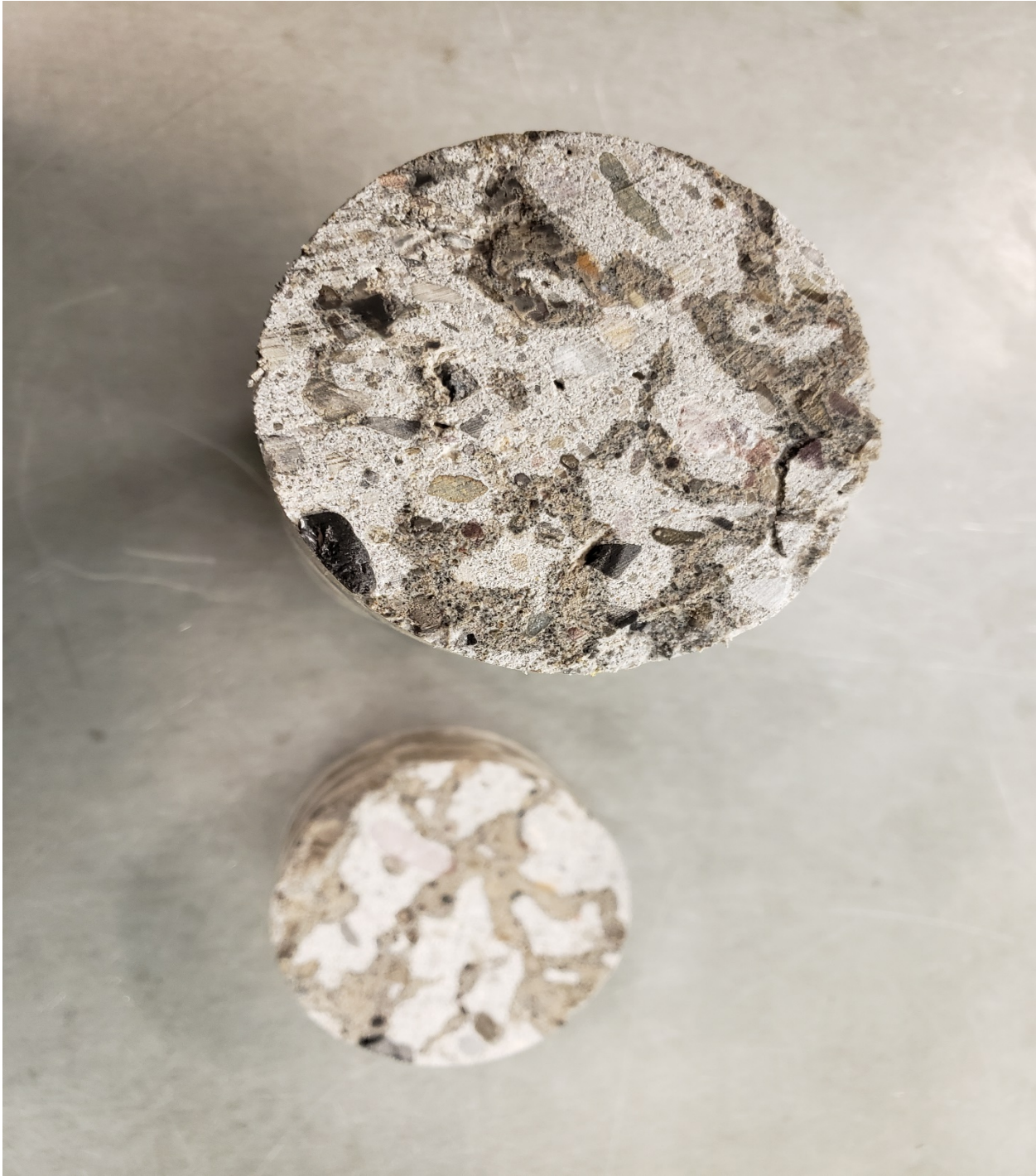
Moisture throughout Core #5 After being Cut
