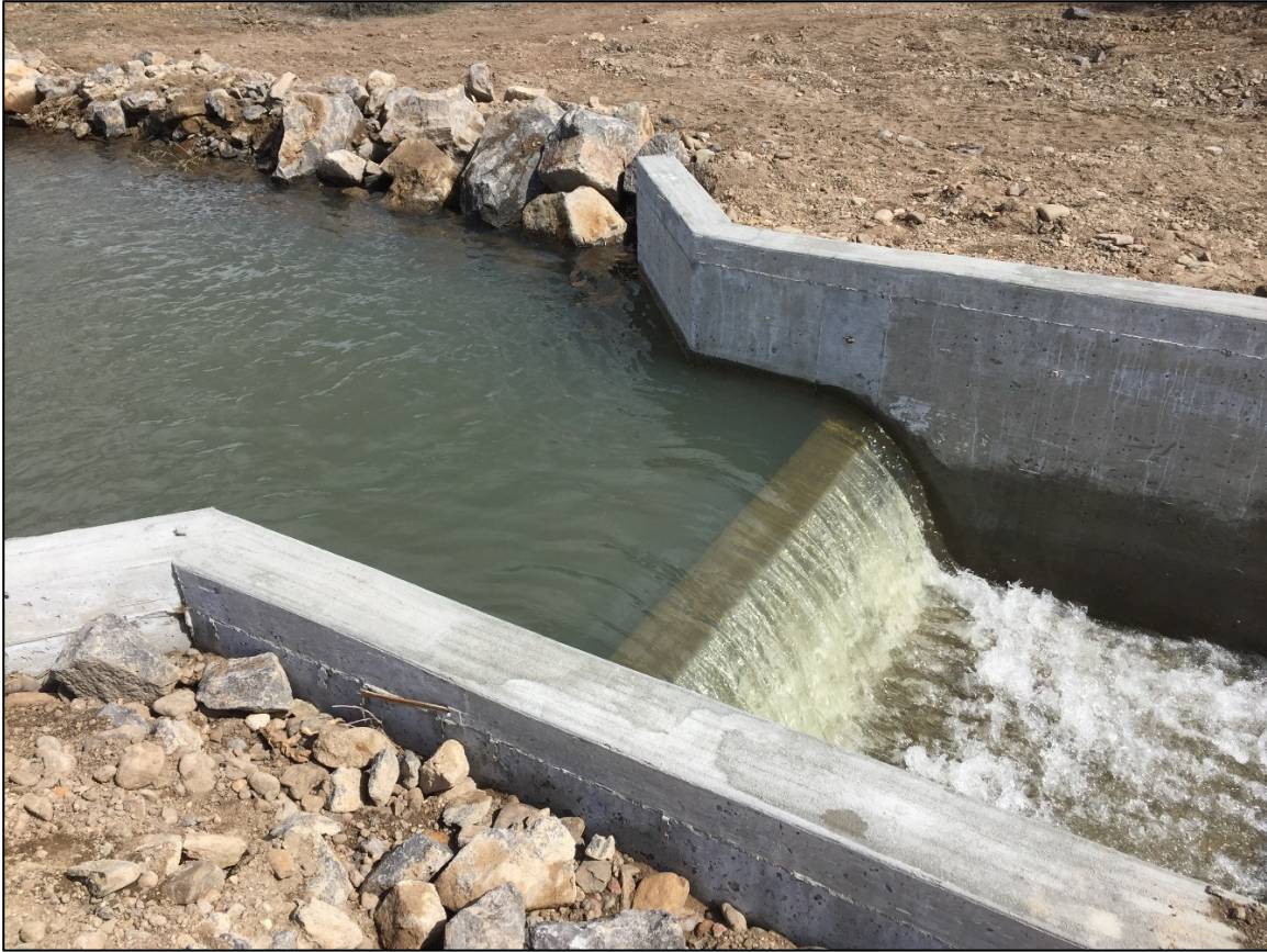
Figure 5. 8-foot suppressed weir at BLM Pit
